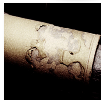
Failed Coating due to undercorrosion
